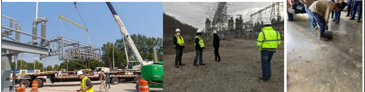
(L to R - just a few pictures of customer visits in recent weeks) - Jobsite at an Ohio IOU, jobsite at a Pennsylvania IOU, drilling demo at public power customer in Kentucky
